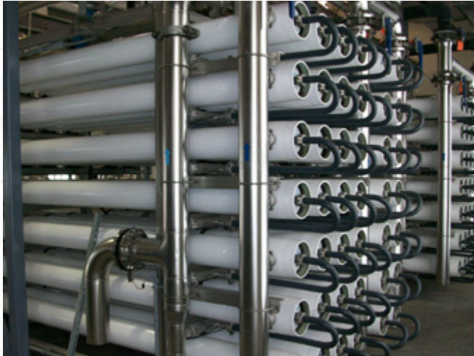
Nanofiltration Water Treatment Plant
