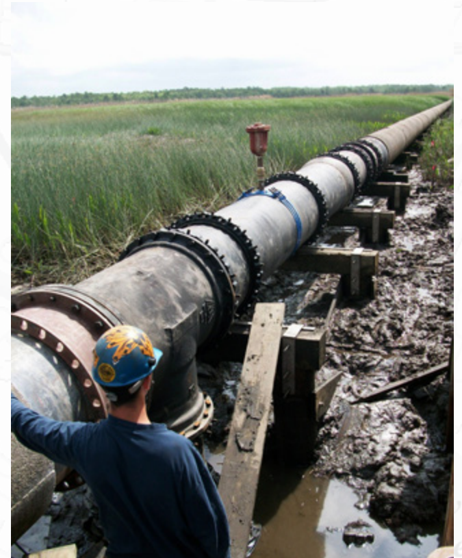
Raw Water Supply Main
