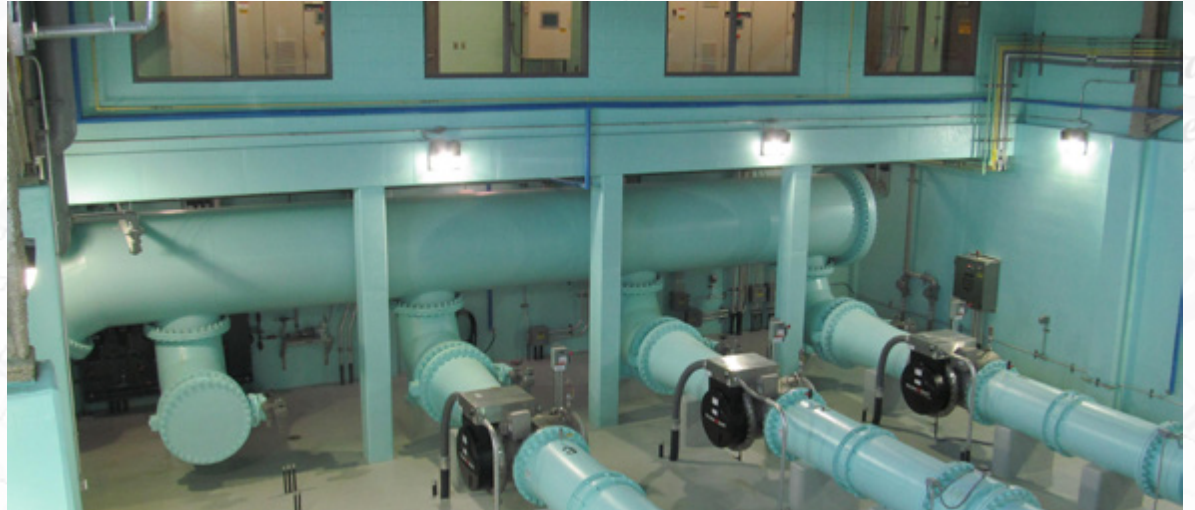
UV Disinfection, Sweeney Water Treatment Plant
