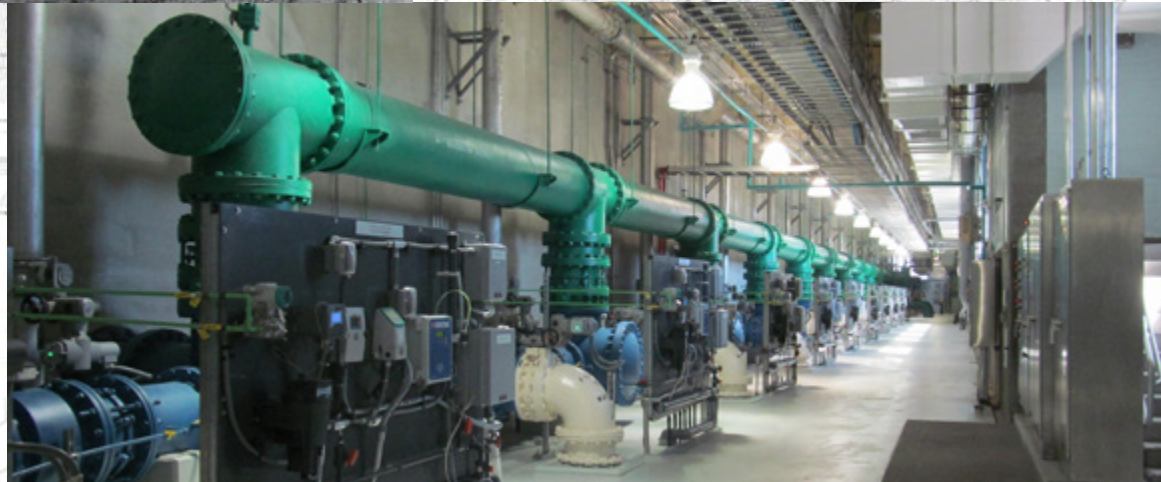
Sweeney Water Treatment Plant, 2016
