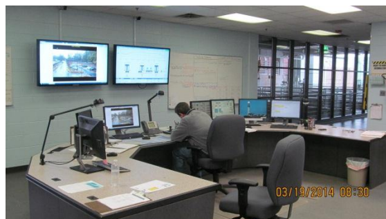
Photographer: Sam Yarboro, Sweeney Water Treatment Plant
