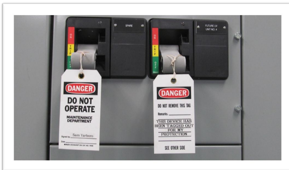
Photographer: Sam Yarboro, Sweeney Water Treatment Plant
