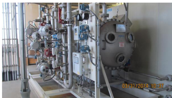
Photographer: Sam Yarboro, Sweeney Water Treatment Plant
