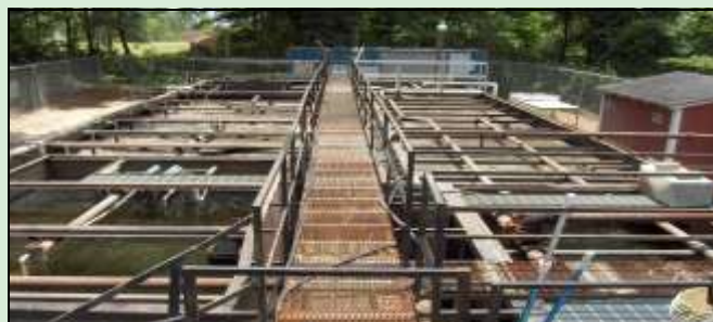
Walnut Hills Wastewater Treatment Plant Permit No. NC0039527 ORC Carol D. Shidal (910) 512-9481
