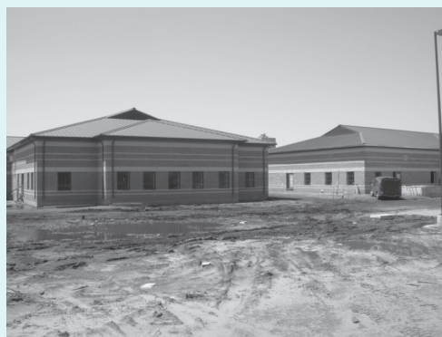
CFPUA's new state-of-the-art nano-filtration plant, located in northern New Hanover County, will be online and ready to serve customers by fall 2009
